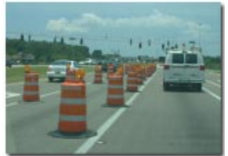
Overpass replacement at U.S Highway 301 and Interstate 75 will cause delays until the end of July.
